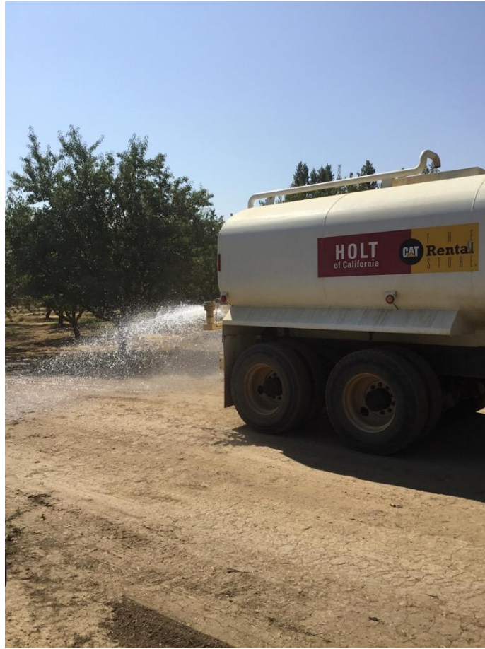
Photo 3: Water truck running to suppress dust during work at Bogue Sub-Line Segment Pole 4/35 in accordance with APM AQ-1.
