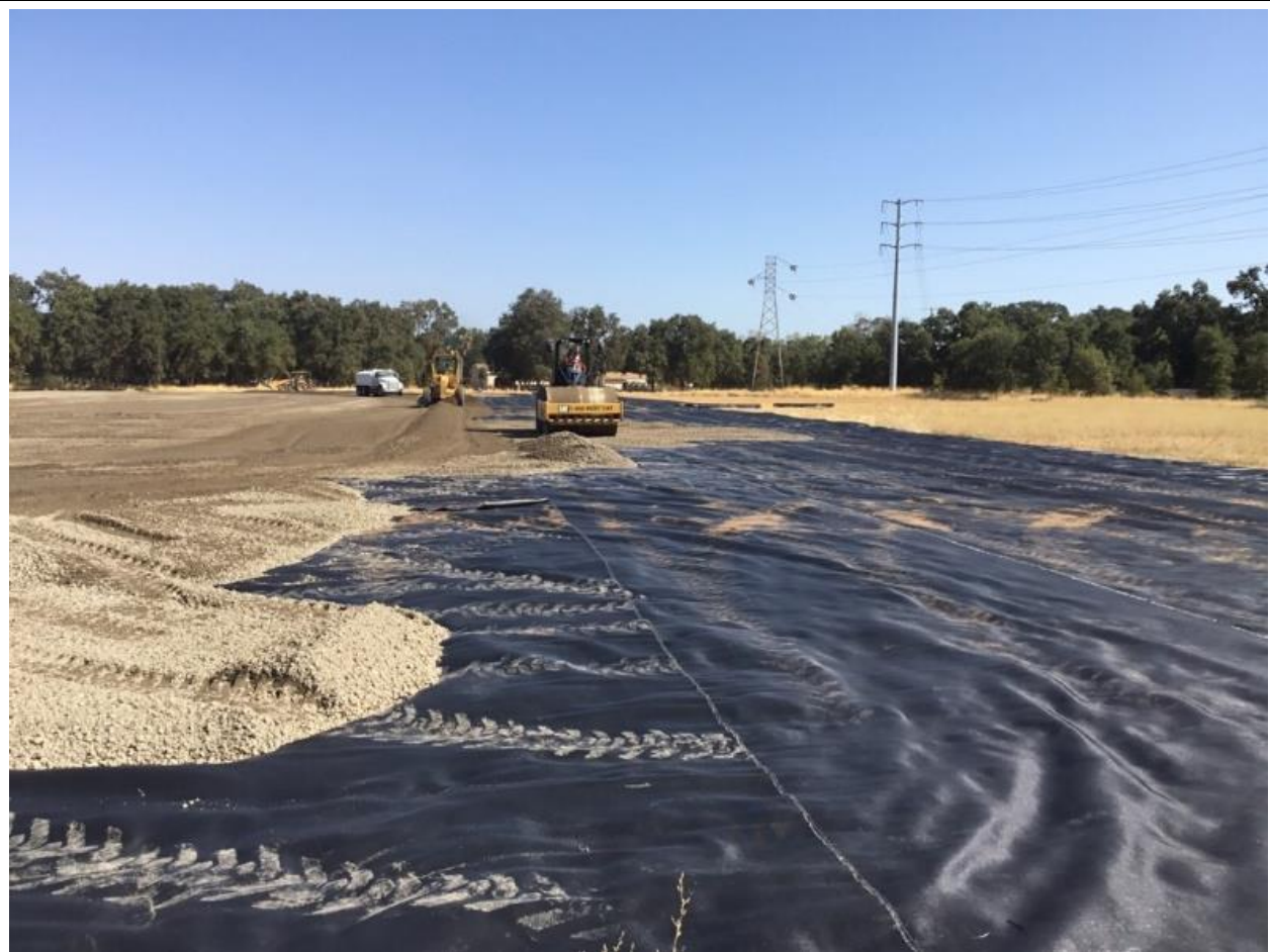
Photo 4: Haul trucks bringing in and compacting gravel to complete winterization of landing/pull site for future reconductoring work at Bogue Sub-Line Segment LZ 4/31.
